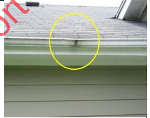
Sagging gutter with evidence of overflowing
