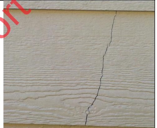
Isolated cracked lap siding
