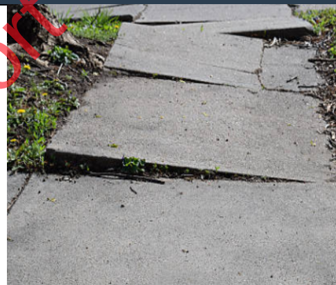
Location of most significant movement due to tree roots
