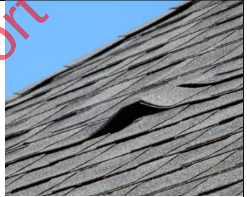
Isolated shingle lift
