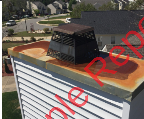
Rust at metal chimney cap with poor drainage
