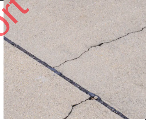
Detail view of cracks
