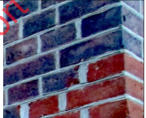
Previous brick replacements evident
