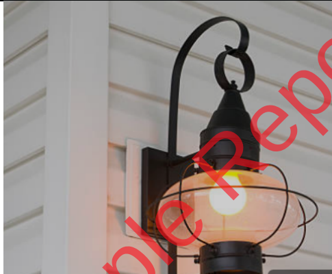
Wall sconce near front door
