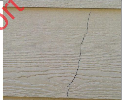
Isolated cracked lap siding
