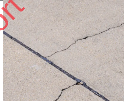
Detail view of cracks
