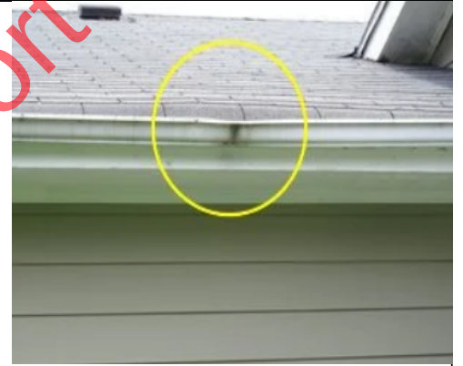
Sagging gutter with evidence of overflowing
