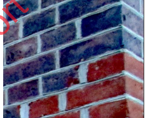
Previous brick replacements evident
