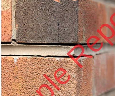
Isolated detached mortar
