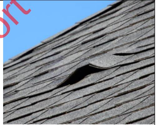
Isolated shingle lift
